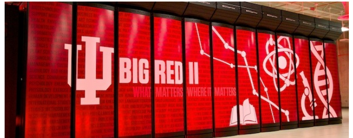
Figure 1: Big Red II in the IU data center.
