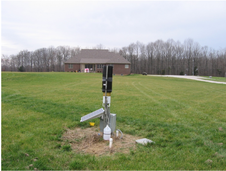
Figure 8. Photograph of above-ground equipment installed at the Control site.
