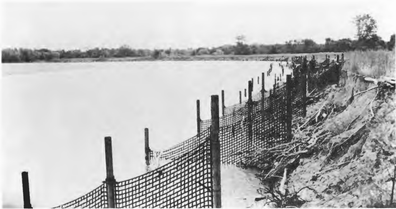
Figure 2. Photograph of part of the east bank of the Wabash River showing permeable jetties installed in 1985-86 by ERCO, Houston, Tex., as preventative of further bank erosion north of New Harmony. Photograph by Shaver (1986).
