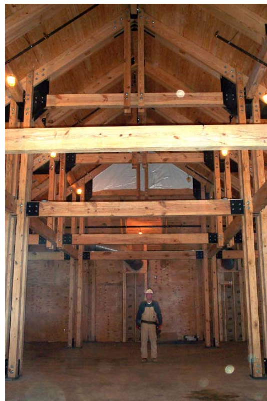
Eighteen years in the making, the Blue Ridge Music Center project nears completion. Photo by Brian Funk, 2005.
